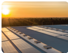
Solar Powered Warehouse Panels
